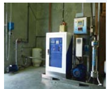
Wairau River Wines, CIP ozone plant
