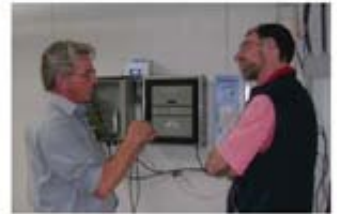
Coolstore gas-phase control elements, Seeka Kiwifruit Industries, Te Puke.
