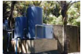
Muriwai township potable water system, fully self-contained design, Rodney DC.
