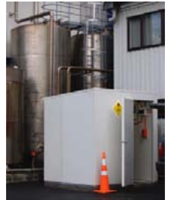
Tip Top CIP factory disinfection plant, Modular design DC-80, Auckland.
