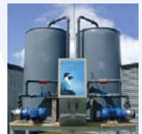
Greenhouse recirculation feed water pathogen treatment system
