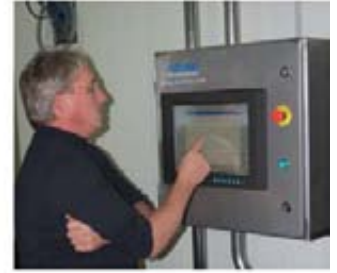
Touchscreen operator interface SCADA water bottling plant, Whakatane
